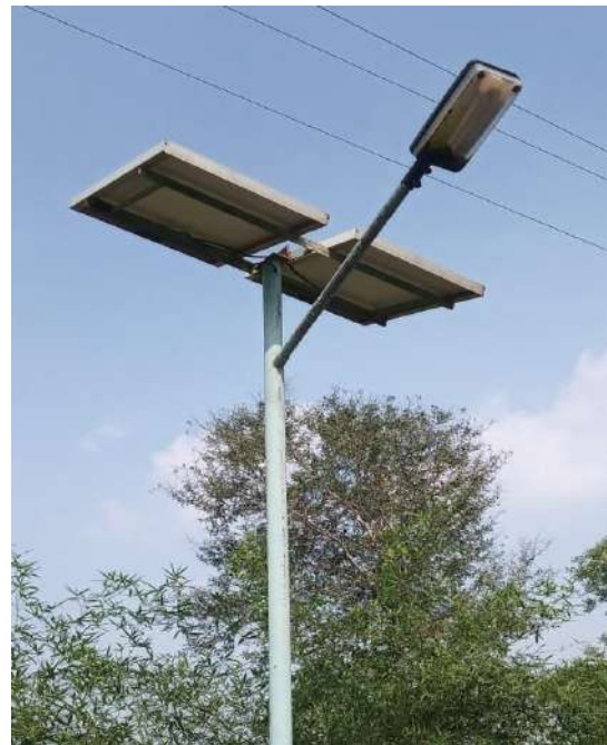
Solar Based Street Lights around College
