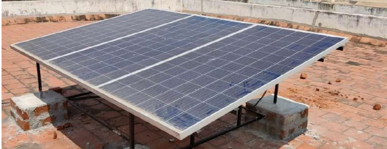
Solar panels in the campus
