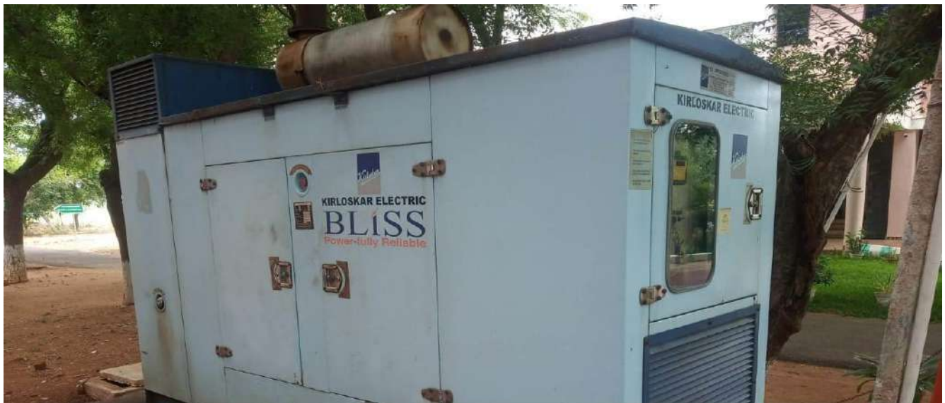
Diesel Generator 125Kva Installed in the College
