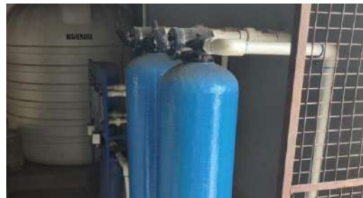
RO SYSTEM INSTALLED IN CAMPUS
