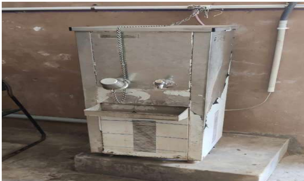
Purified Water Unit Installed In all Blocks
